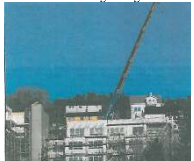
Becoming a block of flats: One after another, the modules are being put in place in the block of flats.
